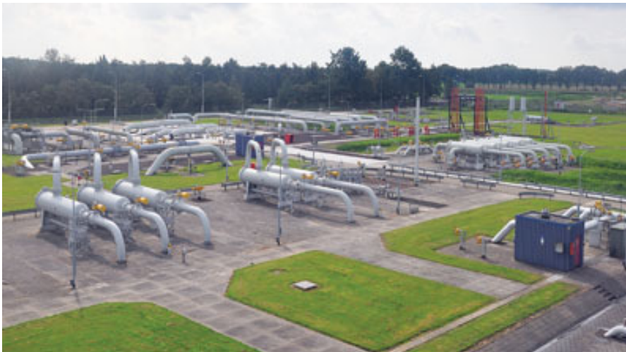
Gas treatment installation
